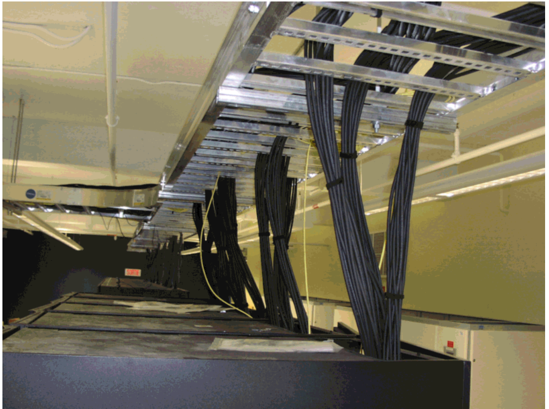
Figure 1-8: Cable Bundles between Leaf and Core Switches
